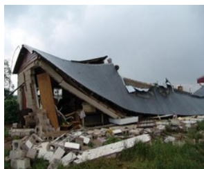
Damage from an EF1 tornado. CASA graduate student Patrick Marsh (University of Oklahoma) conducted a damage survey to verify the EF1 tornado identified in CASA data. Credit: CASA.
